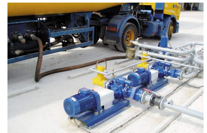
Truck loading (Heating Oil)
