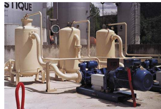
Caustic soda Transfer
