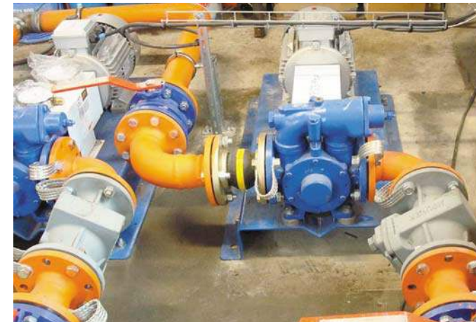
Heating Oil transfer
